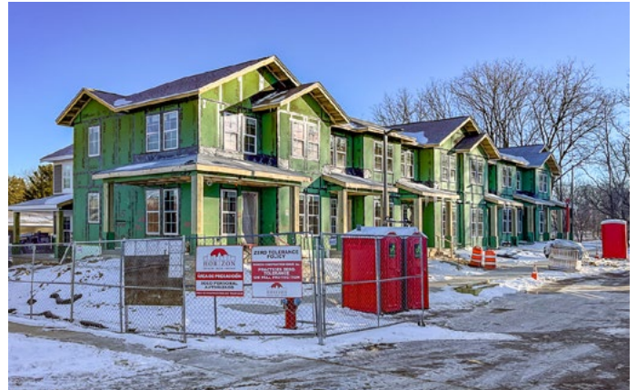
Figure 3: These townhomes under construction on Ellis Potter Court off of Schroeder Road will house families, but are part of a larger affordable housing development by Horizon Development Group and JW Realty Investments with financial support from the City. The development will include homes reserved for families, older adults, veterans, people with disabilities, and people who have recently experienced homelessness.
